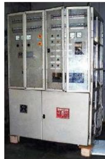
Electronic control panel (Switchboard cabinet)
